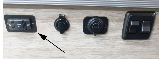
House/Coach Battery Disconnect Switch (Located near sliding door)
