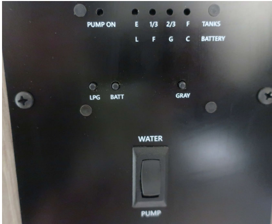
Systems Monitor Panel (Model 59P Shown) -Typical view
