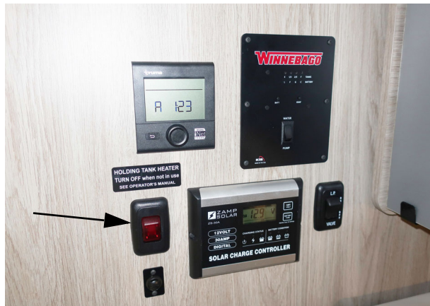
Holding Tank Heater Switch (Located near monitor panel) -Typical View
