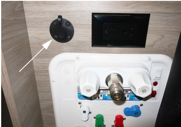
Single Solar Port (Located inside rear door) -Typical view
