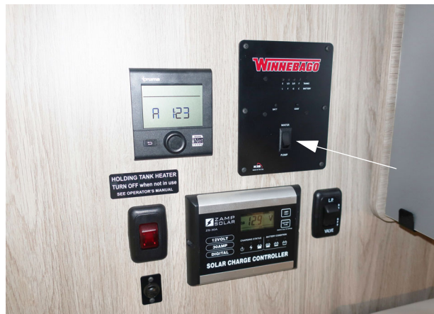
Water pump switch location on Systems Monitor Panel -Typical View
