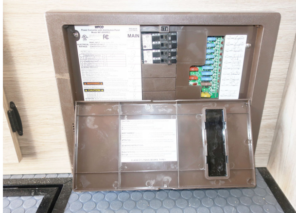
120-Volt Circuit Breakers -Typical View
