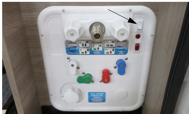
Pump switch -Typical View
